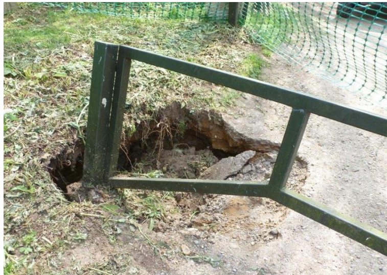
Figure 3: Sink hole at the Vale of Health.
